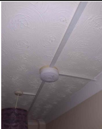
Smoke - Hall (Floor 1)
